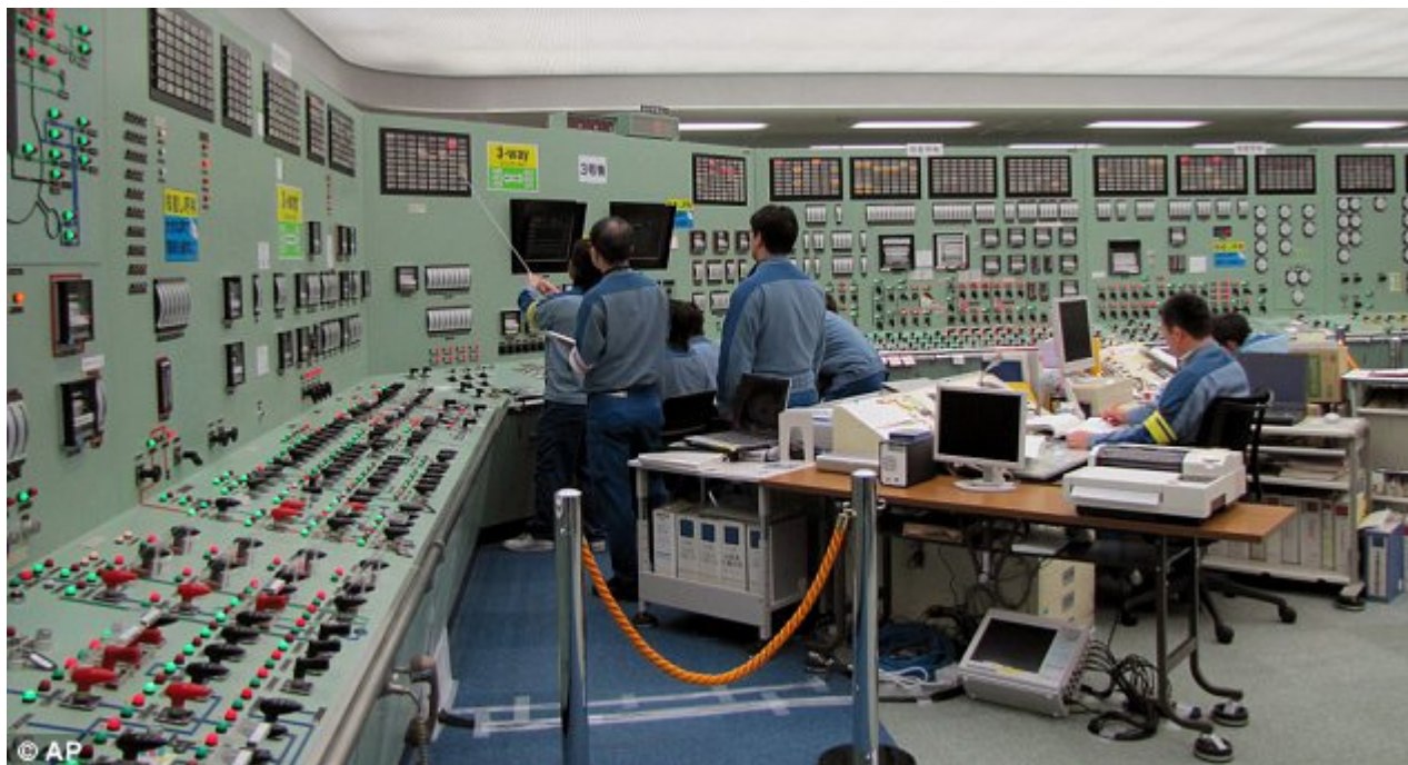
Battling on: Workers inside the central control room of reactor Unit 3 of the Fukushima complex
