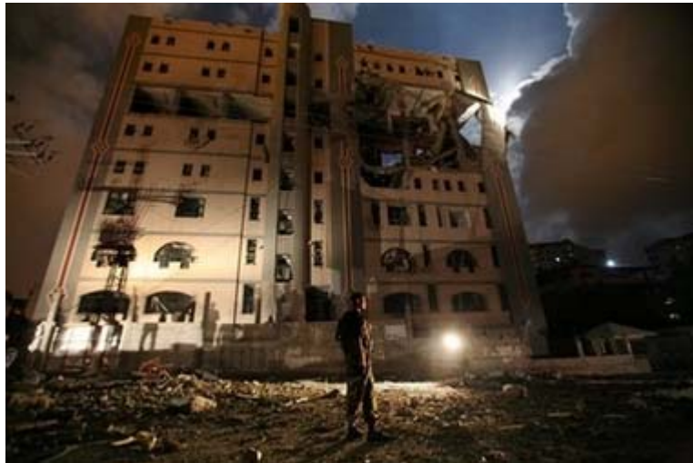
Damage to the Ministry of Foreign Affairs
