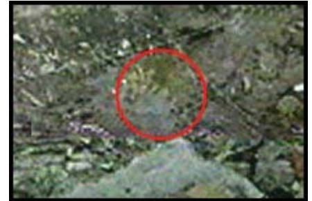
Bottom of crater after slurry was removed with powerful pumps. Sewage continues to leak inside red circle
